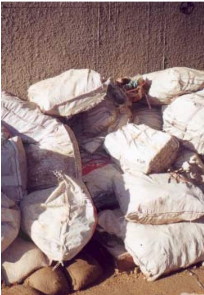
Top: left, improper stacking, right, Improper storage of tiles. Bottom: Improper stacking
