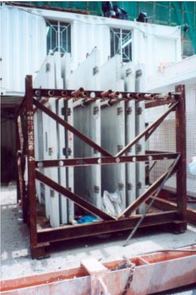
Top: left, packaging waste, right, mixed construction waste. Bottom: Drywall partitions and reusable packaging
