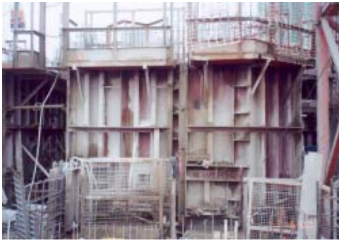
Top: Metal formworks. Middle: left, timber waste from formworks, right, metal temporary work. Bottom: left, reusable platform formwork, right, metal platform work.
