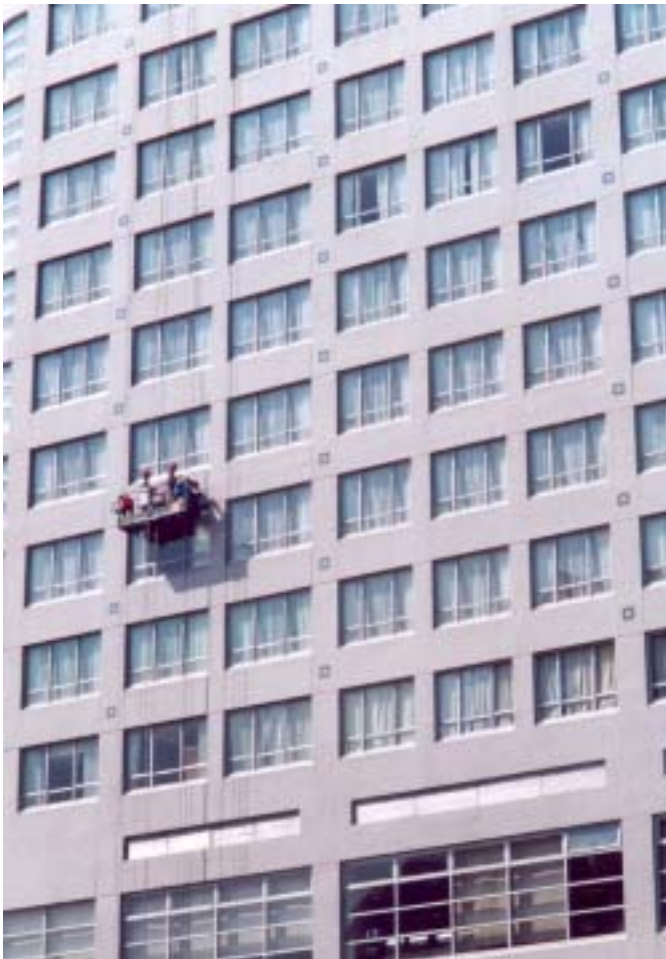
Top: The Hong Kong and Shanghai Bank building maintenance, Central, Hong Kong. Bottom: The YMCA building maintenance, Tsim Sha Tsui, Hong Kong.
