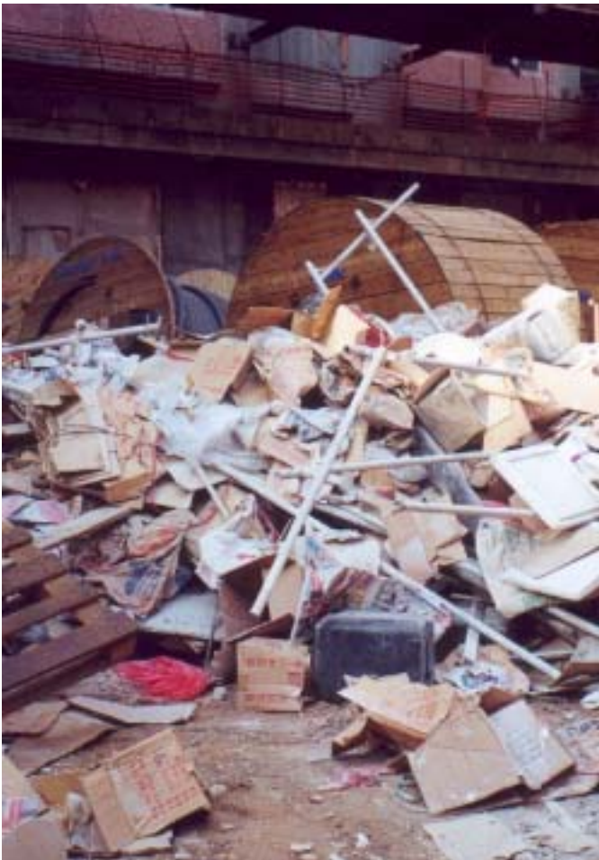
Mixed construction waste
